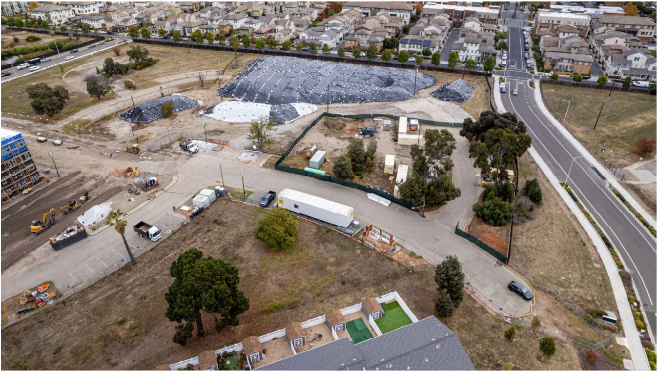
Aerial photo of the stockpile and laydown area. To the left of the photo is corner of the new Mabuhay Street and the future realignment of Lakehurst Circle at the corner of Linnet Corner.
