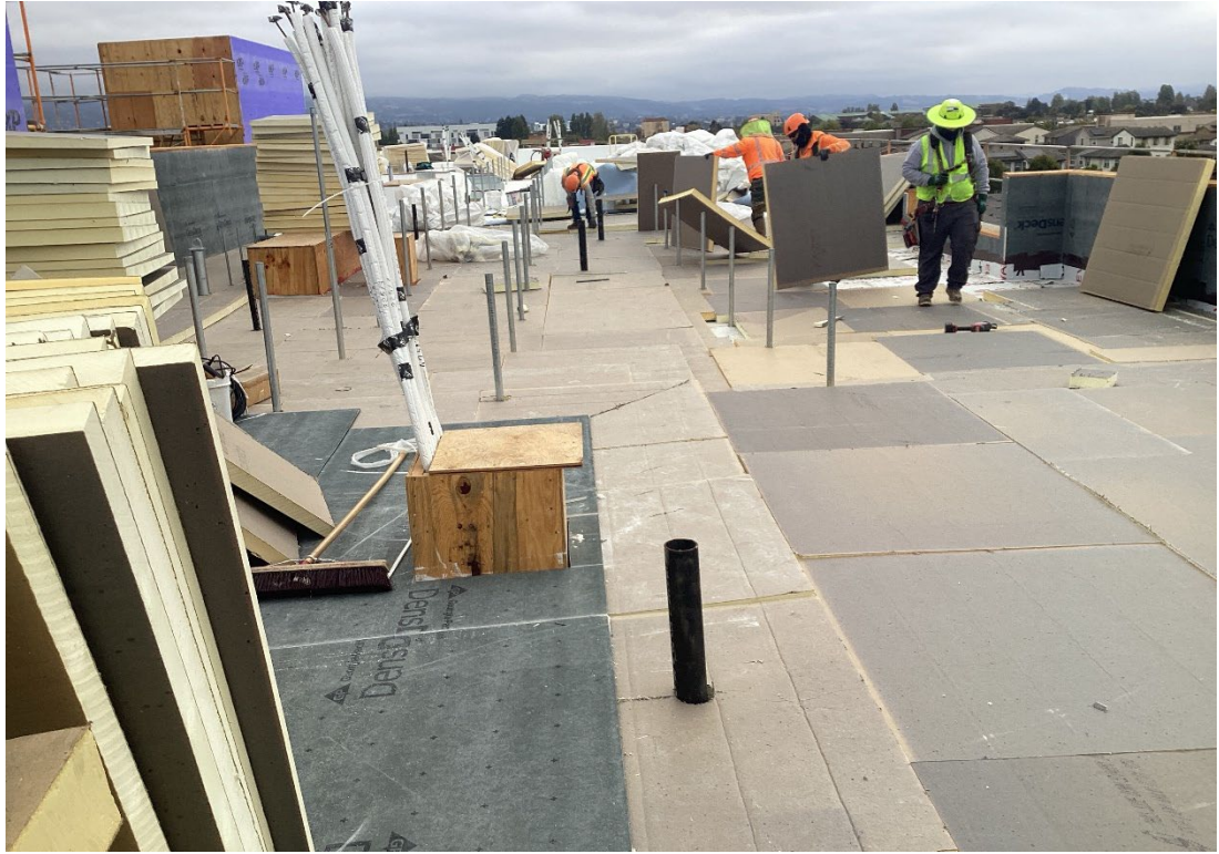
Figure 7: Roof & Exterior Building Maintenance (EBM) Installation
