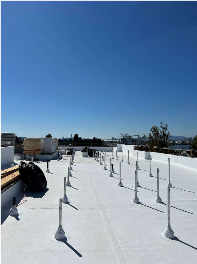
TPO membrane installed on the roof. The white “sticks” scattered across the roof are stanchions to support the solar panels.
