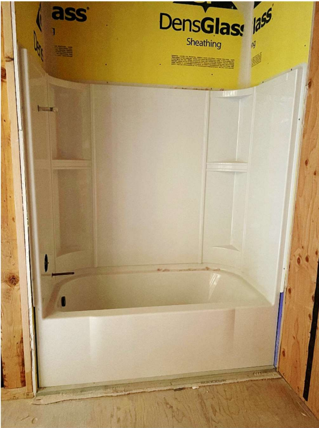
Bathtubs are installed in the units.
