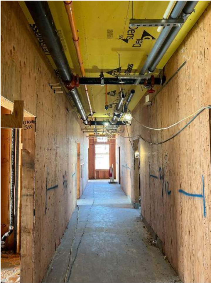
Plumbing lines, water lines, and fire sprinkler system being installed in the hallway.
