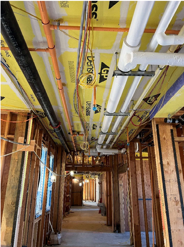
Rough plumbing, rough electrical, and fire sprinkler system installed in the hallway.
