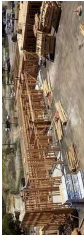
Linnet Corner Will have PV systems
