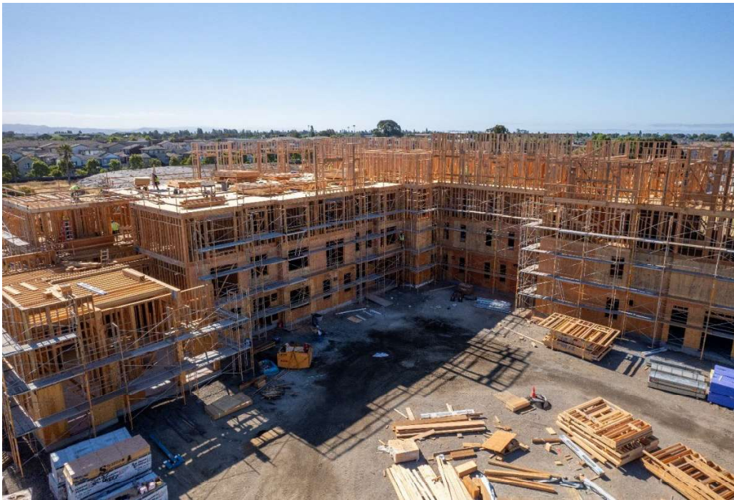
Figure 4: View of scaffolding and framing from parking lot to Linnet Corner's front entrance
